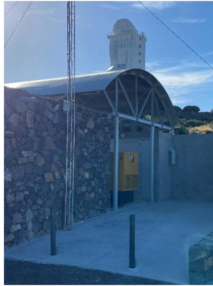
Figure A.3. The transformation center of the ASTRI Array.
