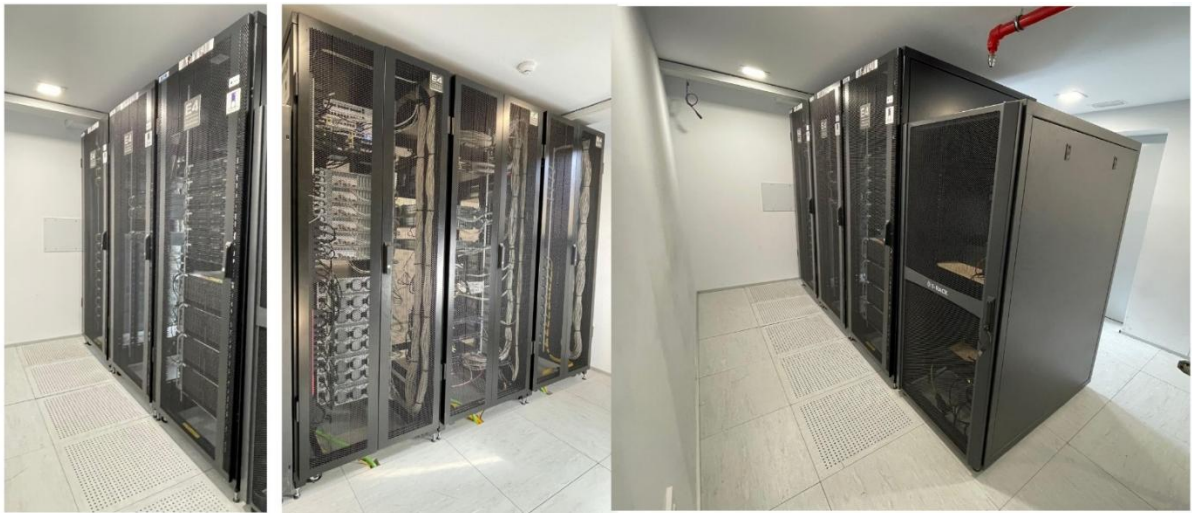
Figure A.9. The ASTRI Array data center in the Teide Observatory Residencia. The smaller rack on the right image belongs to another IAC project.
